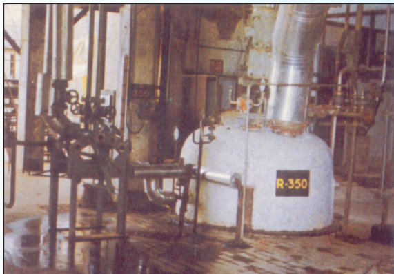
Quinalphos pilot plant developed at NEIST
