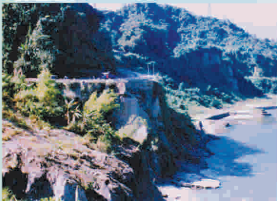
The Landslide prone zone of NH-52(A) at Karshingsa, which is delivering its recorded Big Landslide during July to Sept., 1998
